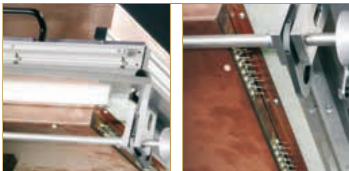
Details of RF shielding
